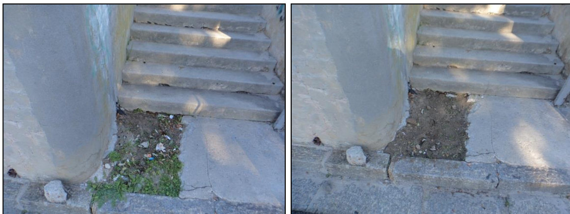
Figure 3: Exposed earth along Alexandra road steps not only presents tripping hazards but also fosters weed growth.
