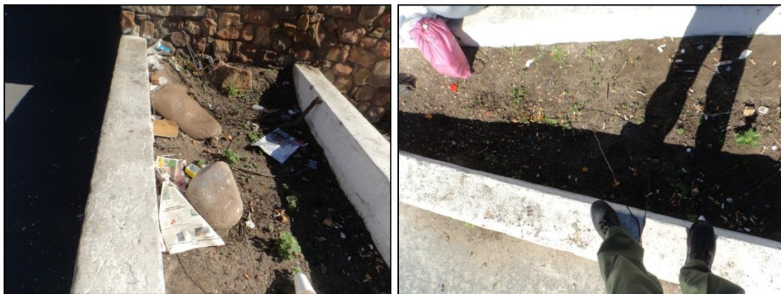
Figure 1: Certain hotspots continue to present problems and the team does their best to address these such as the wall under the Atlantic road bridge.
