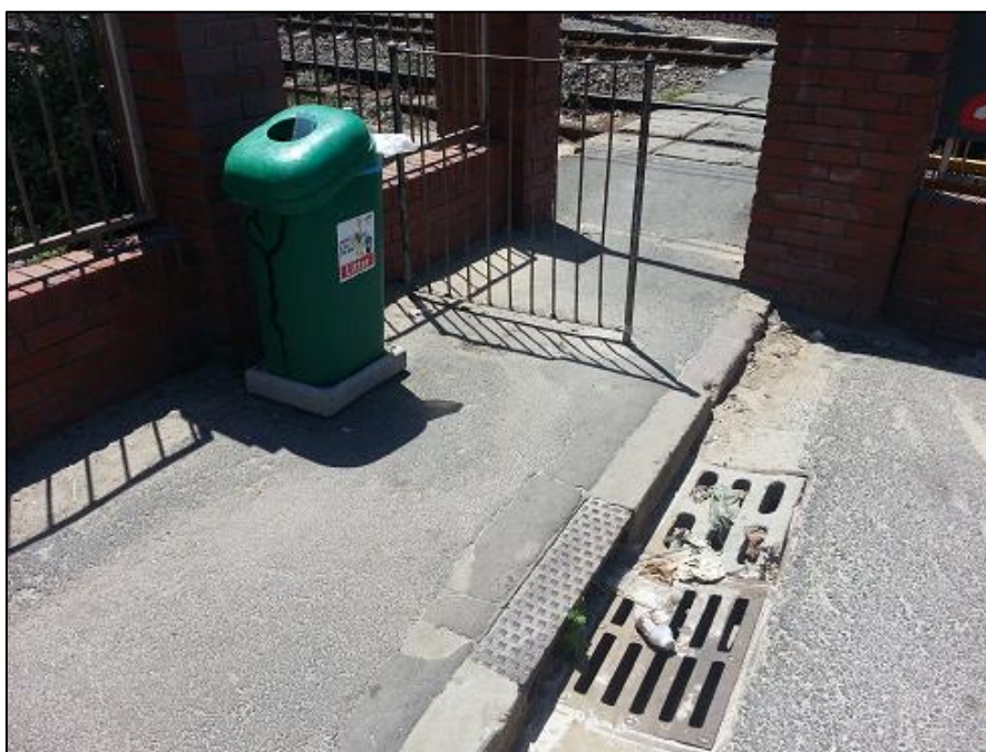
Figure 7: A bin with a broken lid at the railway crossing at False Bay College and a drain being blocked by litter that possibly originated from the bin.
