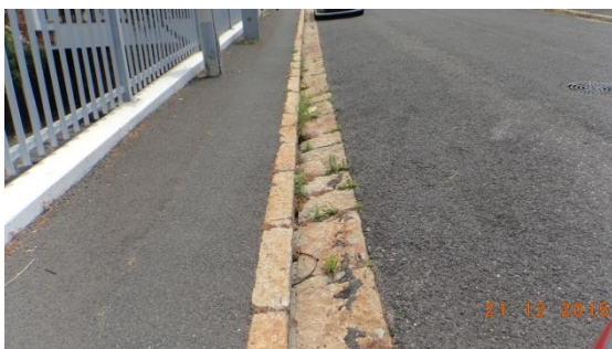
Figure 7.a. Weed filled gutter
