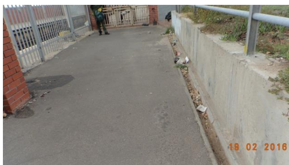
Figure 5.a. Gutters filled with general litter.
