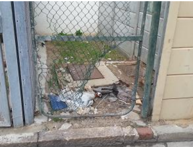
Figure 8: Dumping in the vacant area next to the transformer in Church Street.
