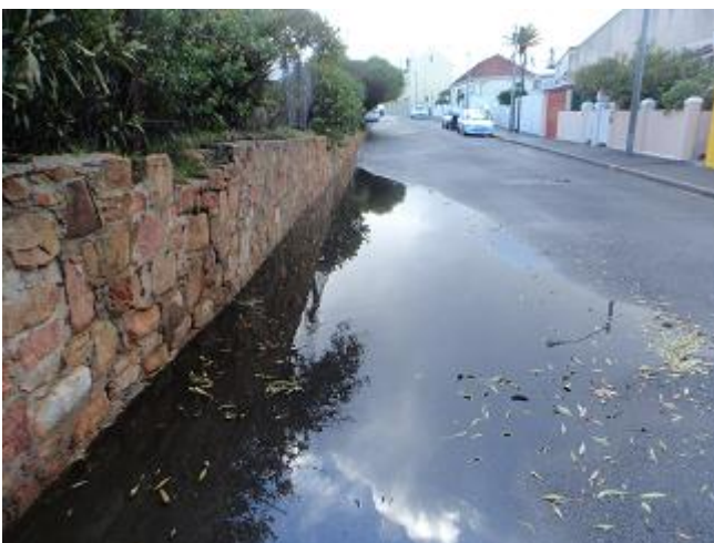
Figure 20: A flooded drain in Milner Road.
