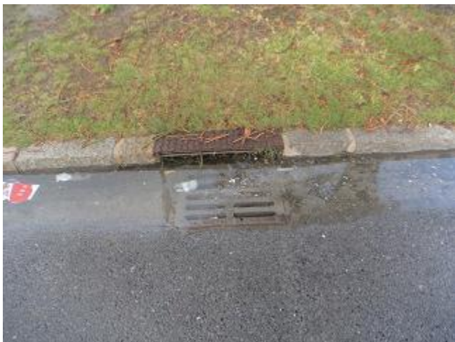
Figure 29: A flooded drain in Royal Road.
