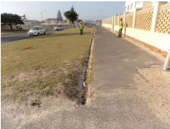
Figure 25: An overgrown gutter filled with sand in Royal Road before being cleaned.
