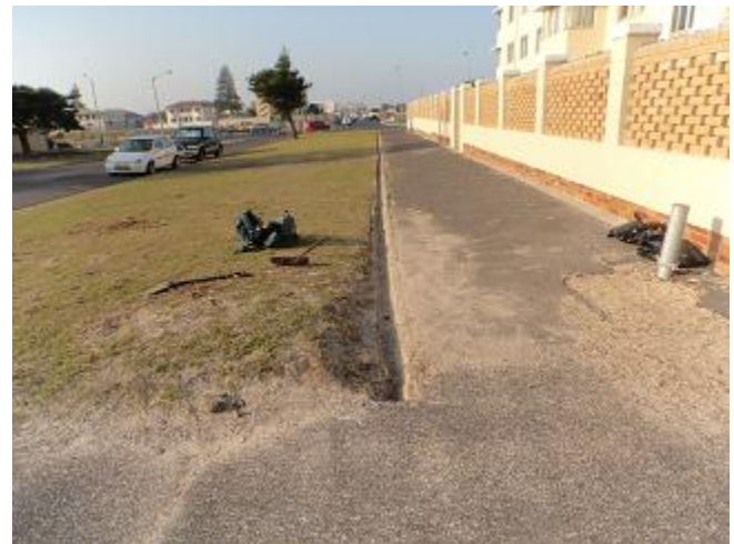
Figure 26: An overgrown gutter filled with sand in Royal Road after being cleaned.
