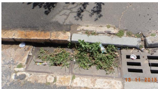
Figure 5.a. Weed blocked gutter
