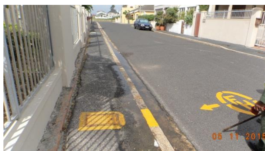
Figure 6.b. Leaking hydrant on Alexander road.
