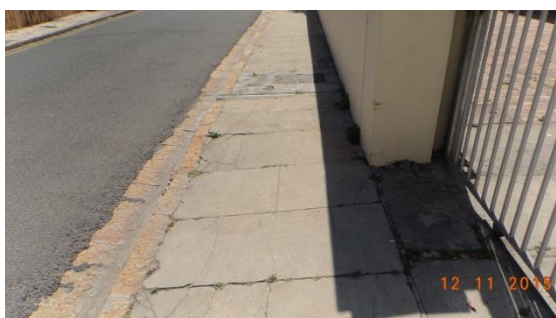
Figure 4.a. Pavement walls showing weeds.
