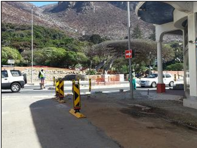
Figure 4: Road Maintenance activities on the corner of Main Road and York Road.
