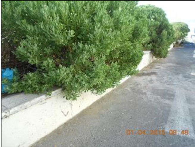
Figure 9: Overgrown vegetation along the railway line in Church Road
