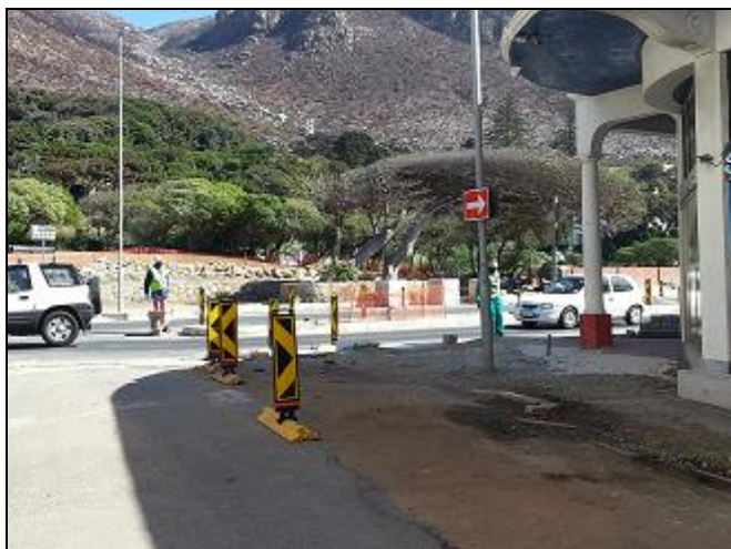
Figure 3: Road Maintenance activities on the corner of Main Road and York Road.
